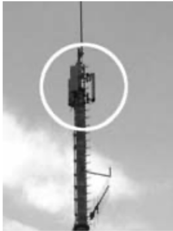
TETRA antenna (very similar to cellphone antennas; three antennas are a characteristic feature).
