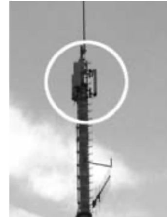
TETRA antenna (very similar to cellphone antennas; three antennas are a characteristic feature).
