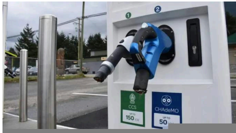
Electric vehicle charging station with severed cables.
